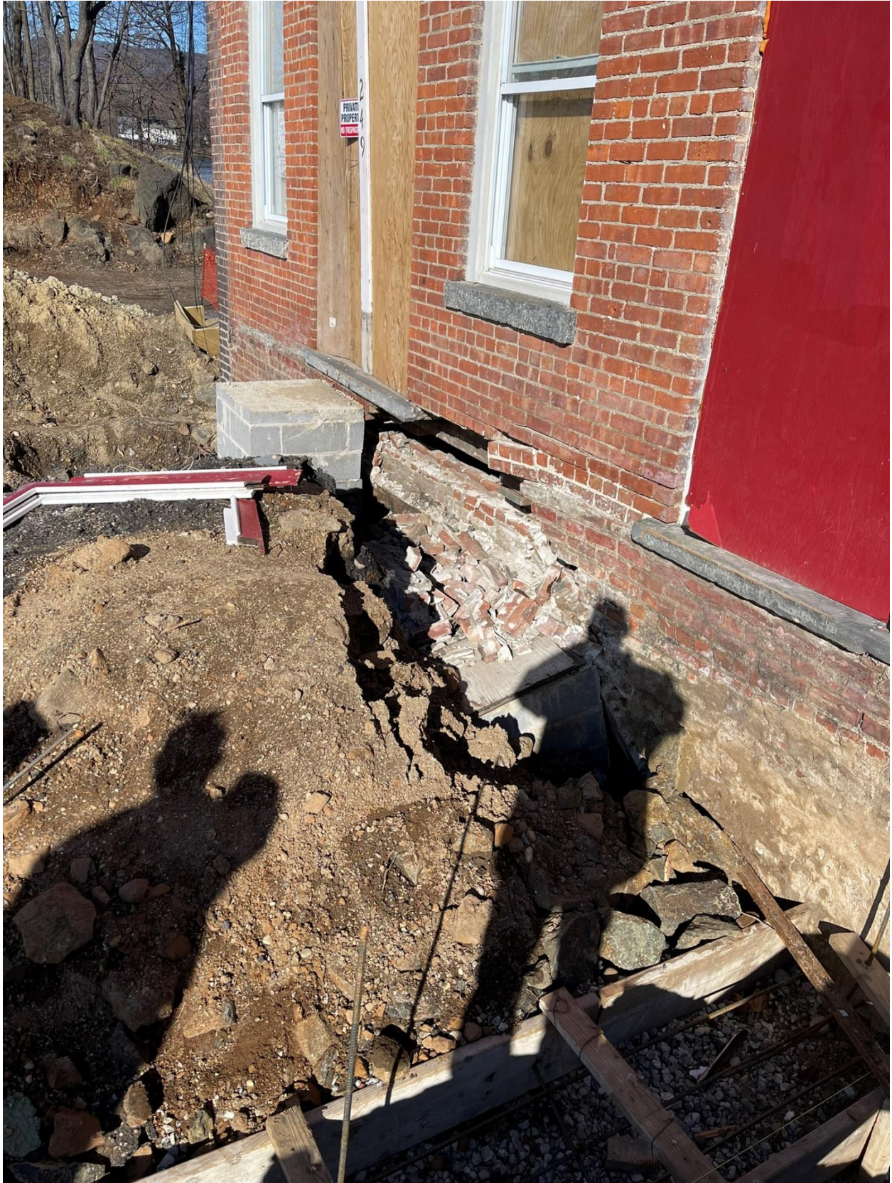
Figure 1 - Front Facade - Foundation Wall Failure
