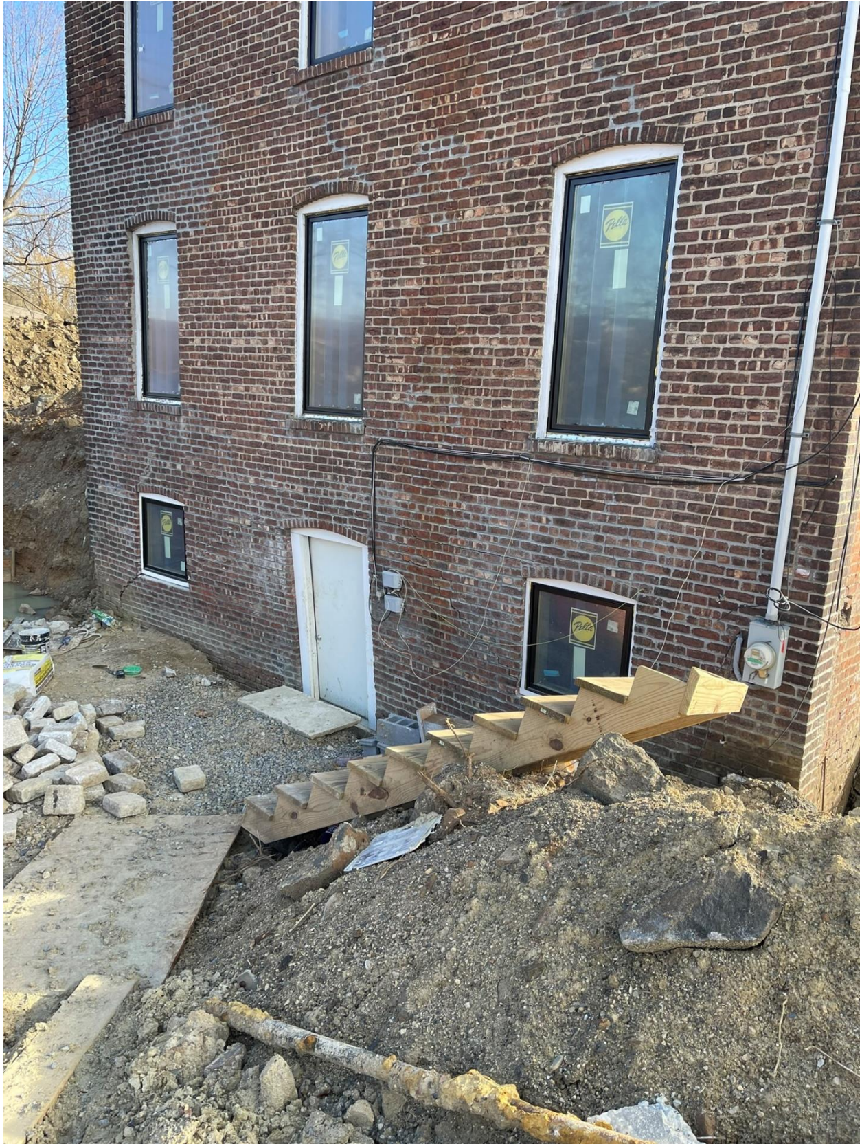
Figure 3 - Foundation Failure of West Facing Facade
