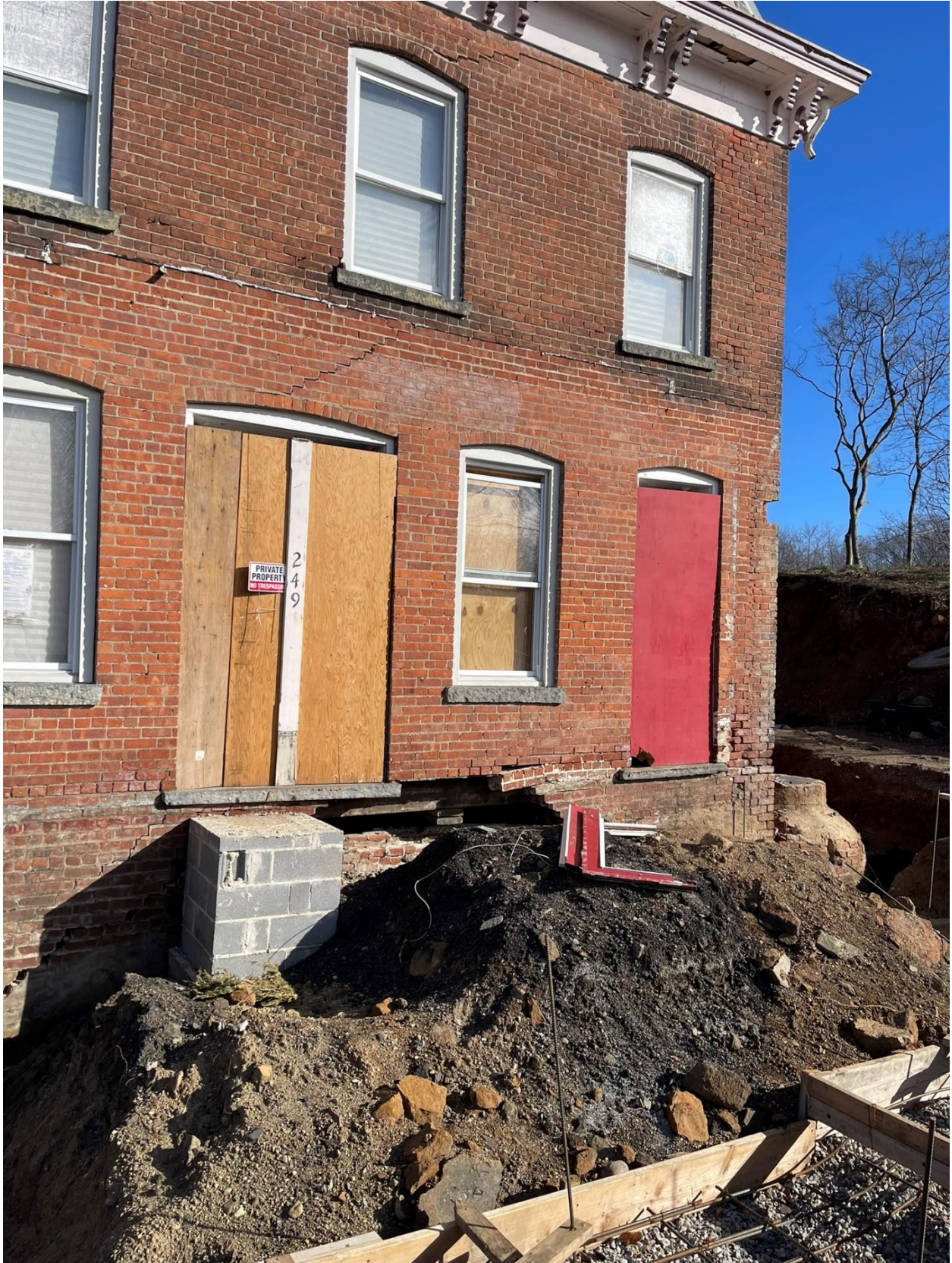
Figure 2 - Cracks in the Front Façade
